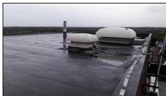
Figure 13: Exhaust duct termination point (Plant Room roof).
