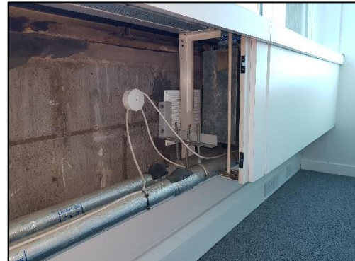
Figure 5: Wall cover removed showing Fan Coil Unit from the side.
