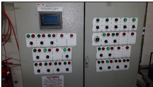
Figure 10: Plant Room control panel.
