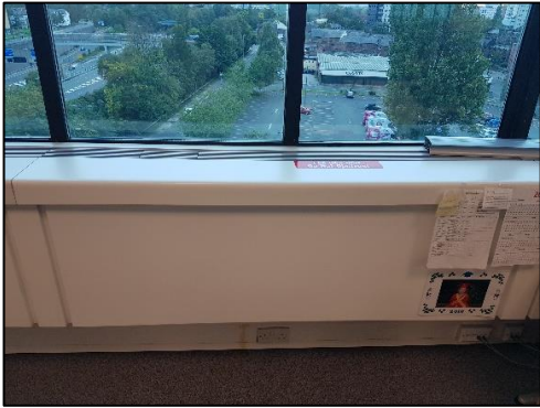
Figure 2: Fan Coil Unit with external cover installed.
