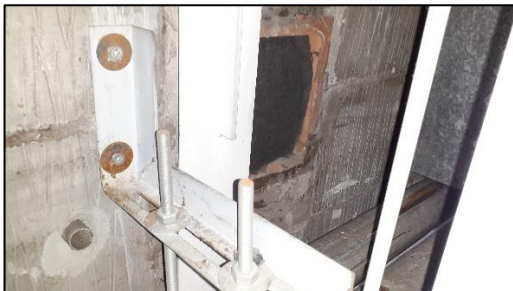
Figure 6: Blocked passive fresh-air vent.
