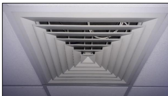
Figure 12: Ceiling-mounted extract grilles.
