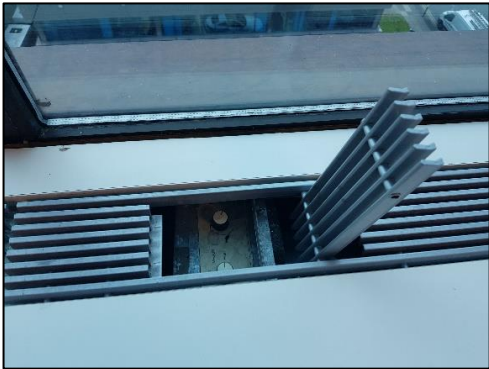
Figure 4: Fan Coil Unit control potentiometers.
