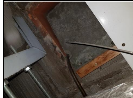
Figure 9: Restricted/obstructed passive fresh-air vent/.
