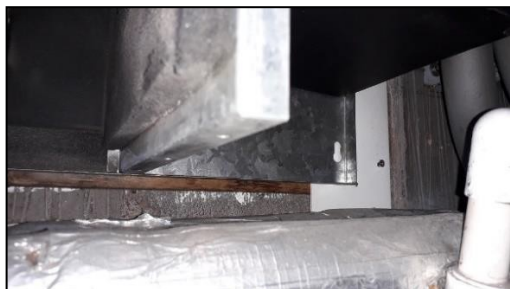
Figure 8: Obstructed passive fresh-air vent due to location of Fan Coil Unit.
