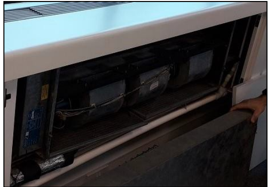
Figure 3: Fan Coil Unit with external cover removed showing motor units.
