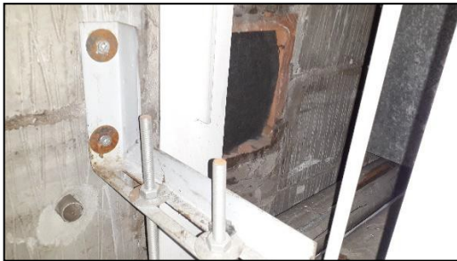
Figure 6: Blocked passive fresh-air vent.
