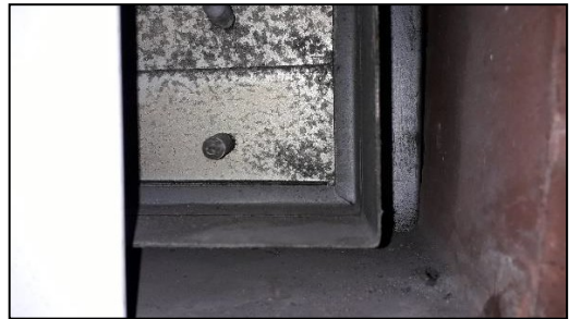
Figure 7: Restricted passive fresh-air vent (dampers in closed position).
