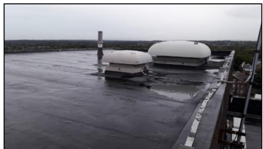
Figure 13: Exhaust duct termination point (Plant Room roof).
