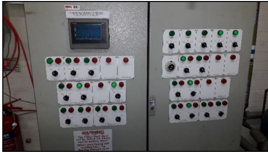
Figure 10: Plant Room control panel.
