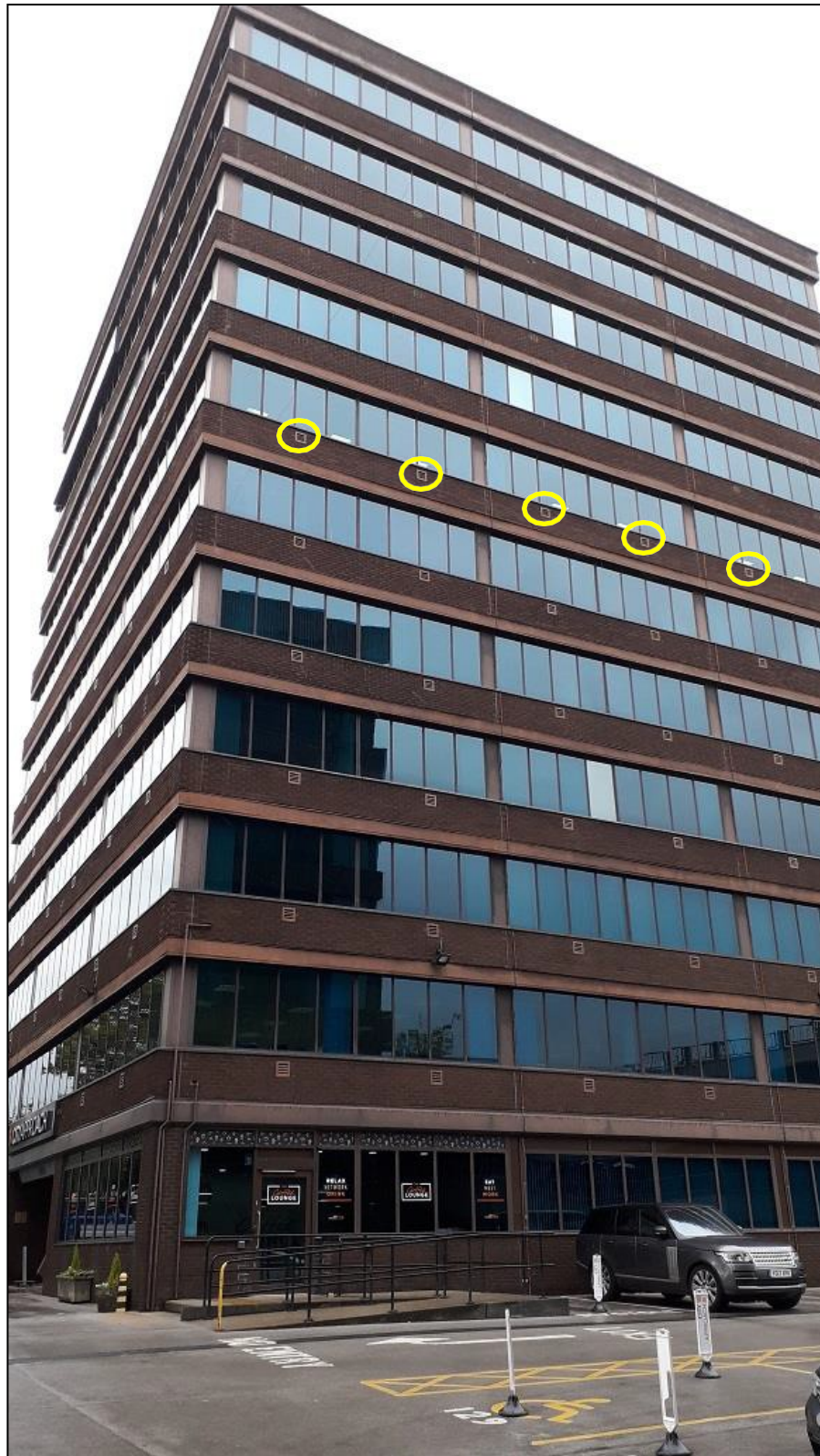
Figure 1: South elevation to 1 City Approach showing five (5) of the twenty four (24) passive ventilation grilles on the 6 th Floor.
