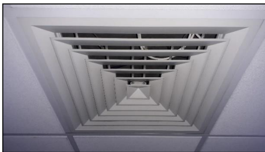
Figure 12: Ceiling-mounted extract grilles.
